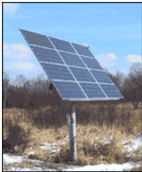
SOLAR PANEL ARRAY
